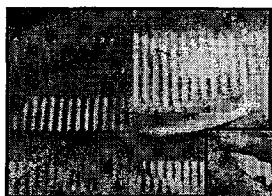
Rear of EF-4 filter - close-up.
